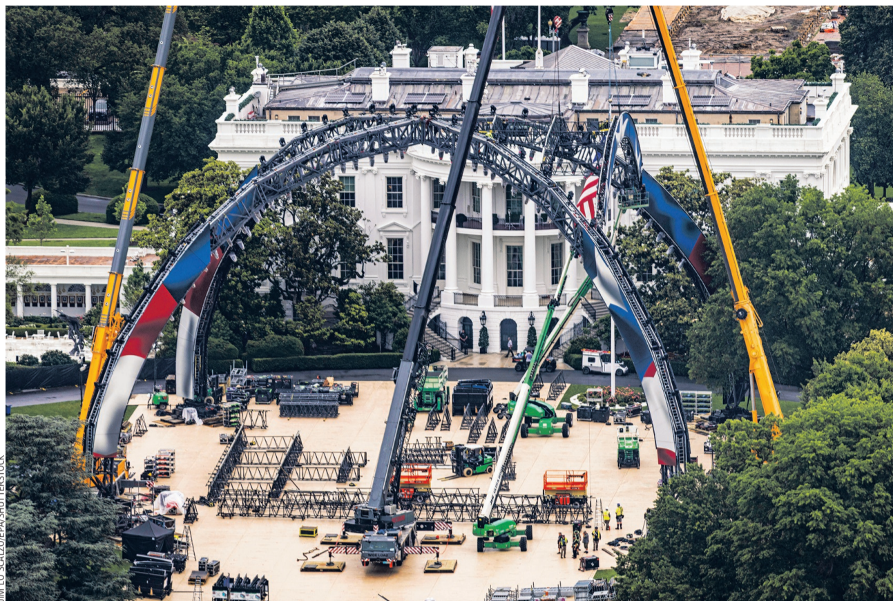
RING OF POWER: Construction was under way Tuesday on a temporary octagon for mixed-martial-arts fights on the White House's South Lawn. Several UFC events are to be staged there June 14, which is Flag Day and President Trump's 80th birthday.
