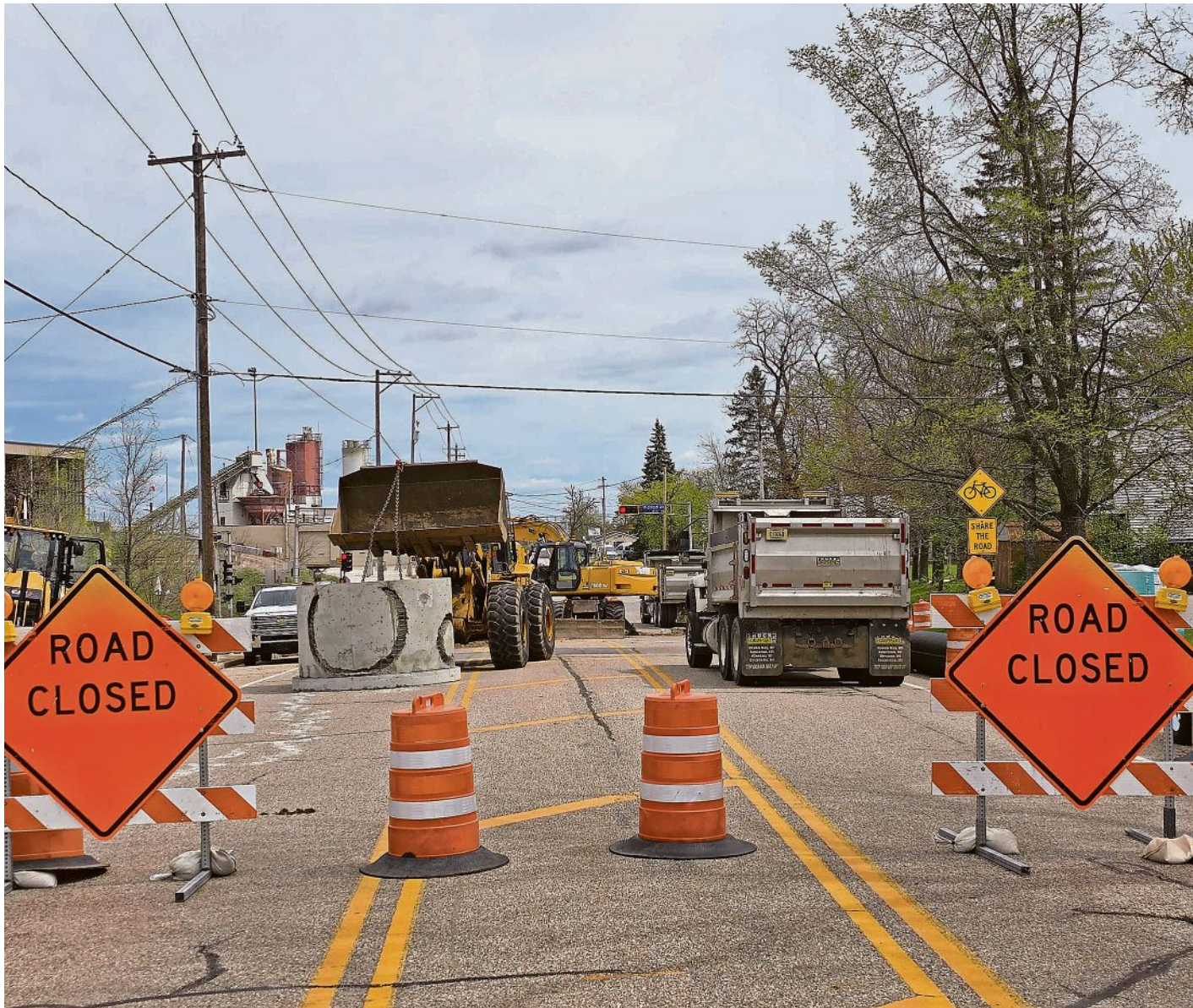
A closure of Patch Street between Blaine Street and Michigan Avenue is expected to last two weeks beginning April 28, 2026 while a parallel storm sewer pipe is installed to help improve drainage in the area. ERIK PFANTZ/STEVENS POINT JOURNAL
