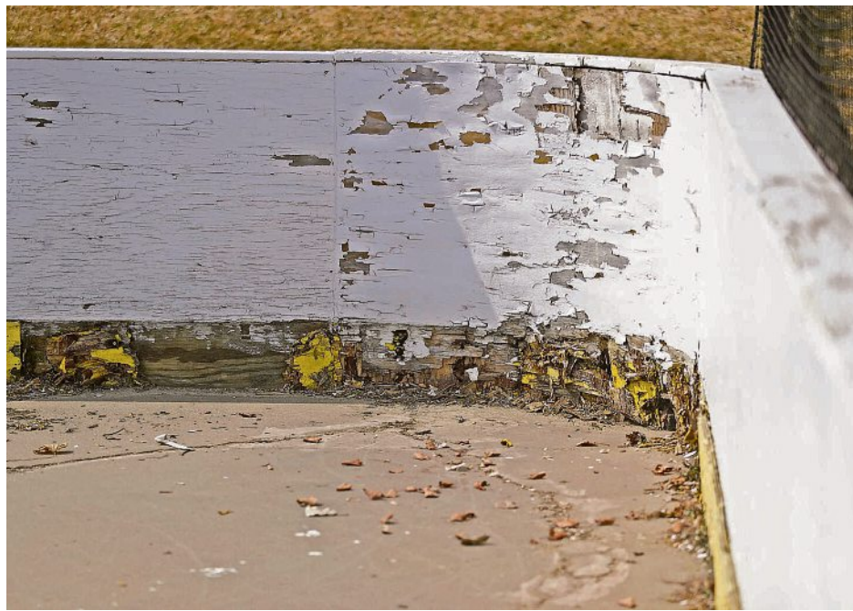
The boards of the roller hockey rink at Patriot Park in Grand Chute are in need of repair or replacement. PHOTOS BY WM. GLASHEEN/USA TODAY NETWORK-WISCONSIN
