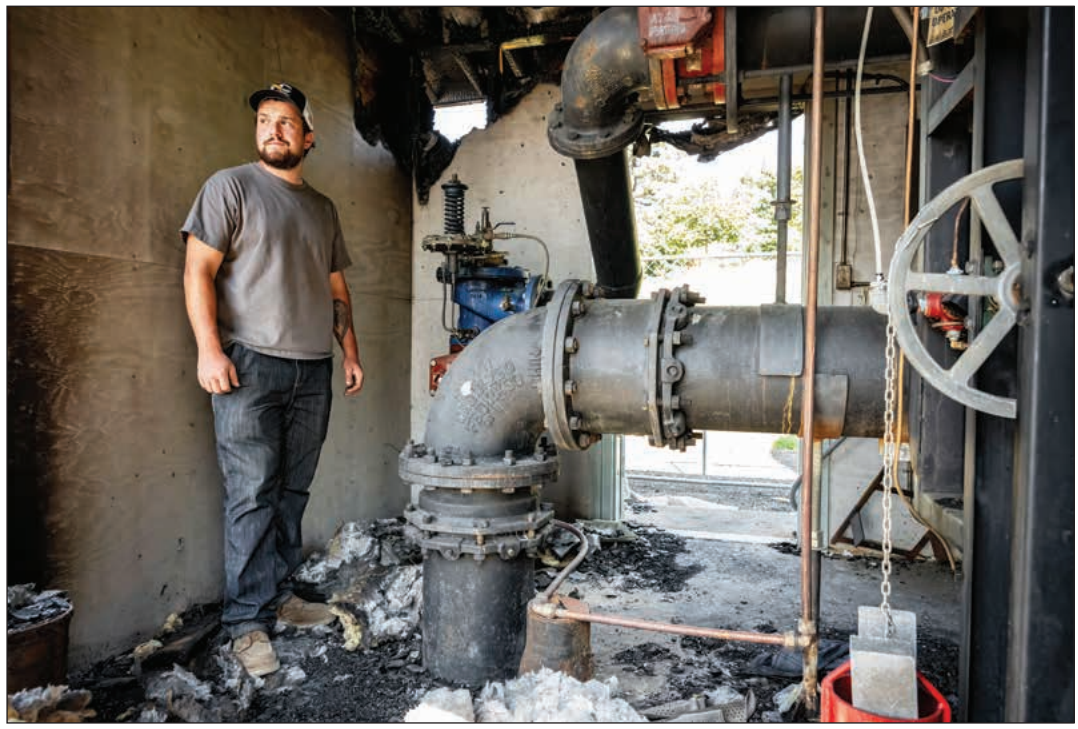
COLIN MULVANY/THE SPOKESMAN-REVIEW Blake Robins, of the city of Spokane Water Department, stands in the valve room of the burnt but still functioning Indian Hills water tank.
