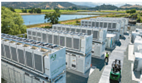
A proposed Chesapeake battery facility, like this one in California, would sit on a portion of a larger 180-acre parcel located about a mile from the Chesapeake Expressway.
