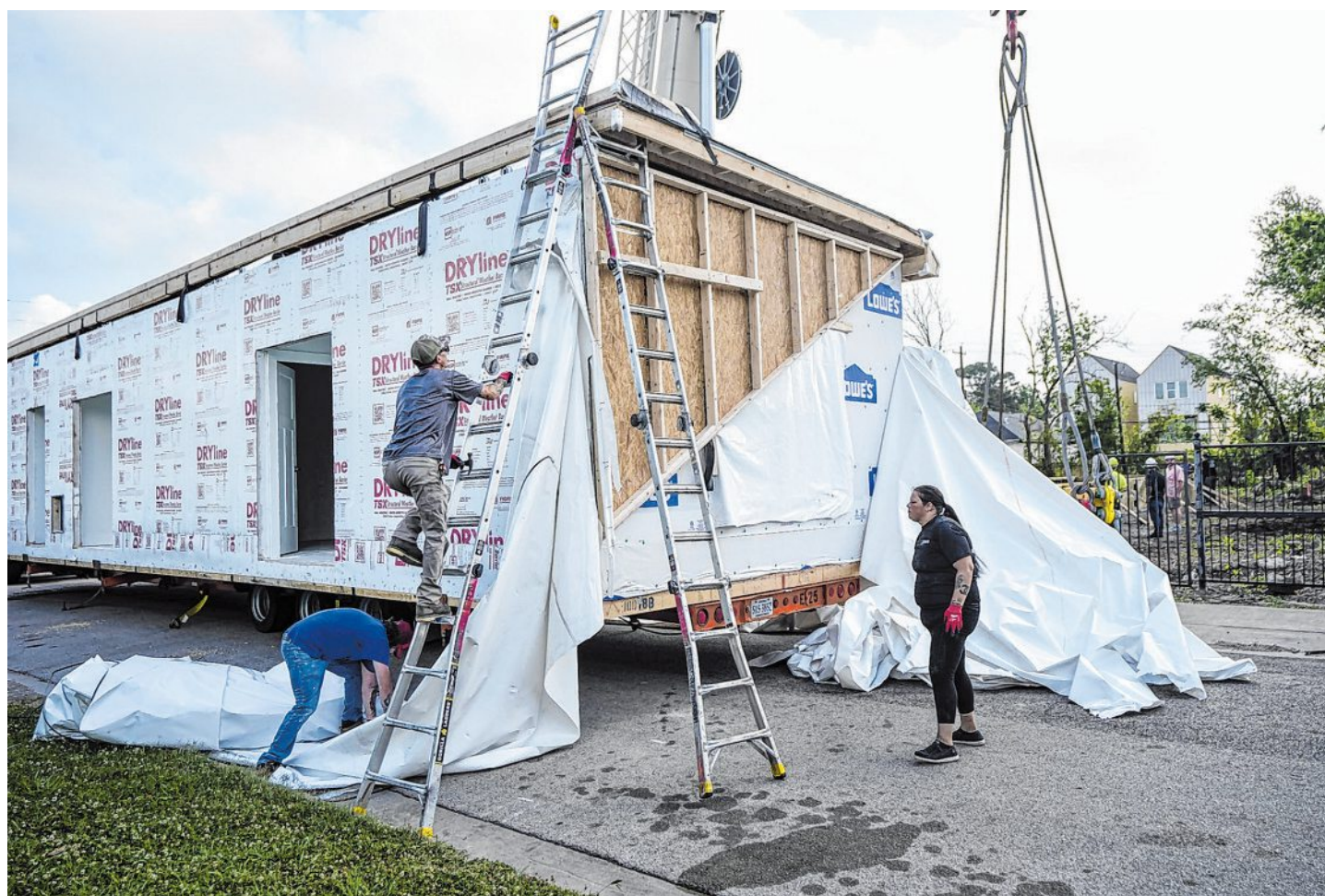
Brett Coomer/Houston Chronicle Workers prepare a Habitat for Humanity modular home to be lifted onto its foundation on March 31 in Houston's Fifth Ward.
