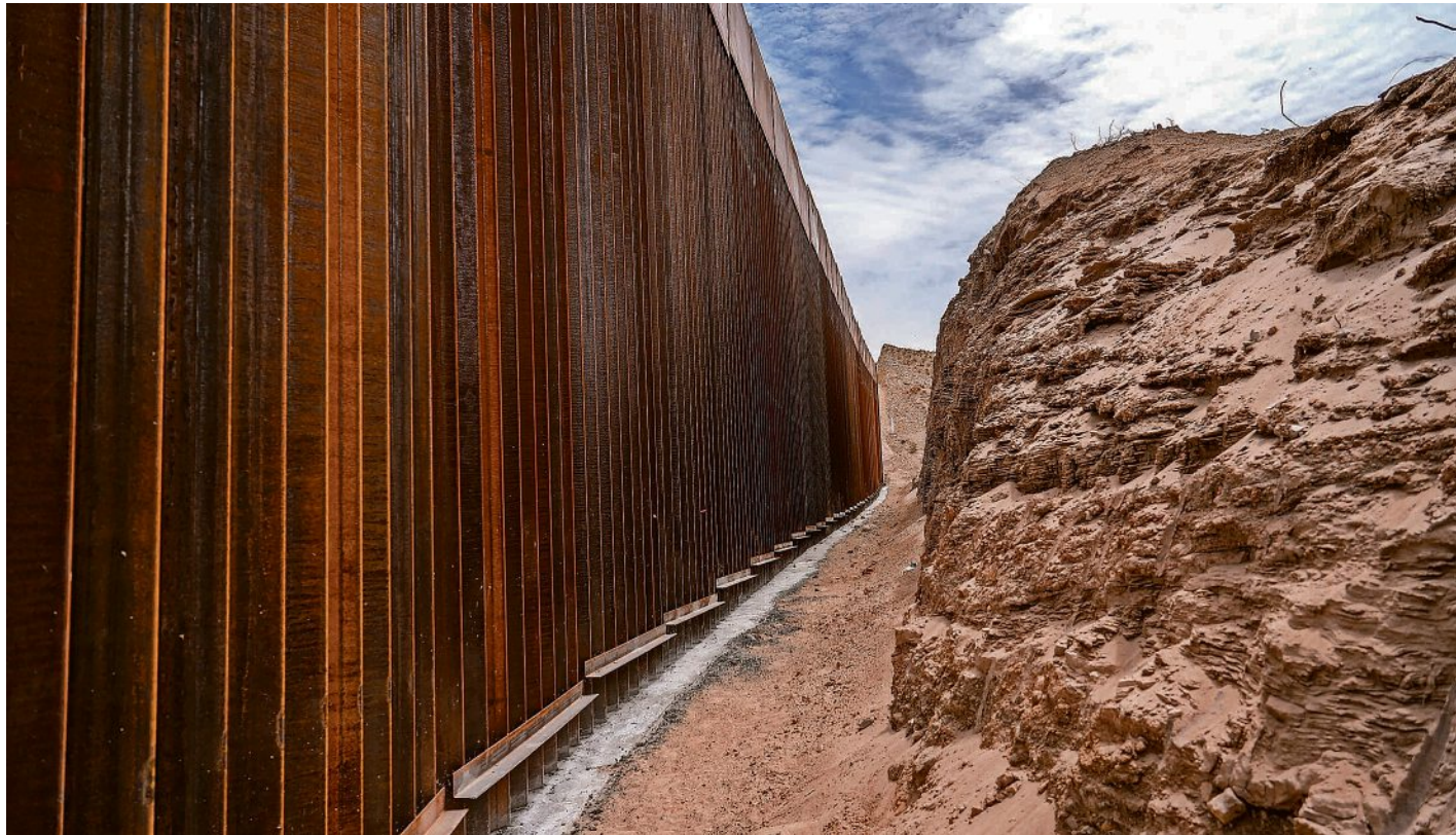
A border wall is seen April 29 where part of the rock was blasted for construction at the base of Mount Cristo Rey as viewed from the Mexican side of the border. PHOTOS BY OMAR ORNELAS/EL PASO TIMES
