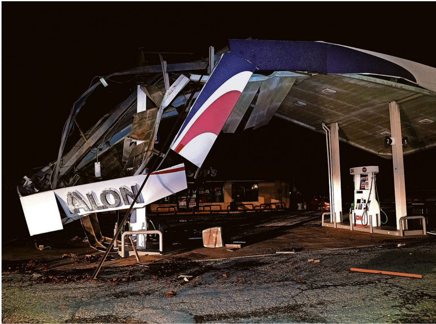
The Allsup's at 765 Veterans Drive was damaged after 75 mph wind gusts swept through Abilene when a severe thunderstorm struck the city Sunday. Much of the city was left without power for the rest of the evening.
