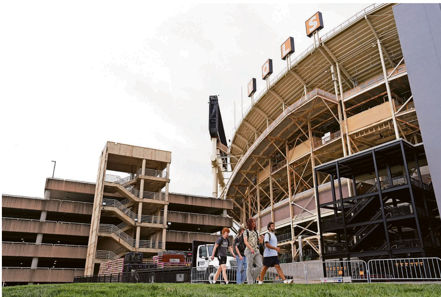
The G10 garage – familiar to many going to events at Neyland Stadium, Food City Center and the University of Tennessee – will be partially demolished this summer, then rebuilt as part of the development of the new Neyland Entertainment District project. CAITIE MCKEIN/NEWS SENTINEL
