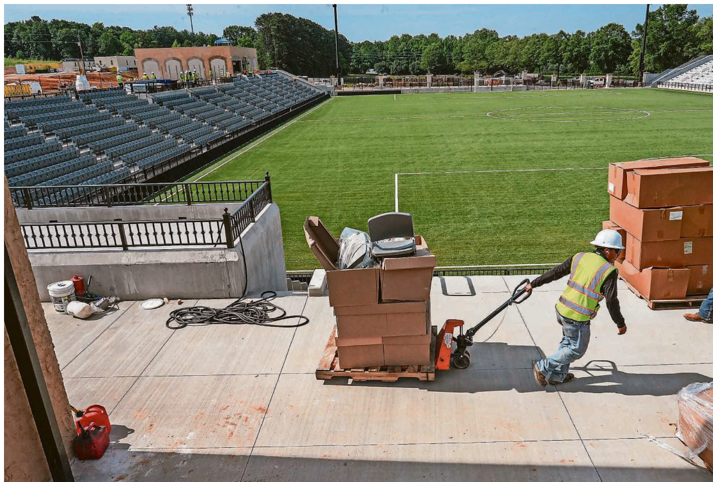
Construction is being finished at GE Vernova Park at BridgeWay in Mauldin on May 29. The first Greenville Triumph game is June 3. PHOTOS BY KEN RUINARD/USA TODAY NETWORK - SOUTH CAROLINA
