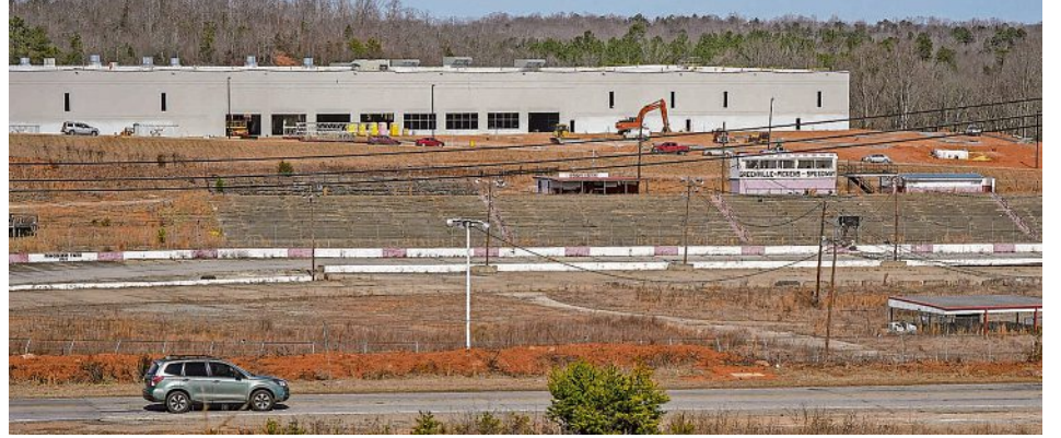
Cars drive along State Highway 123 by the former Greenville-Pickens Speedway and the construction of the Speedway Industrial Park in the city of Easley in Pickens County. KEN RUINARD/USA TODAY NETWORK - SOUTH CAROLINA
