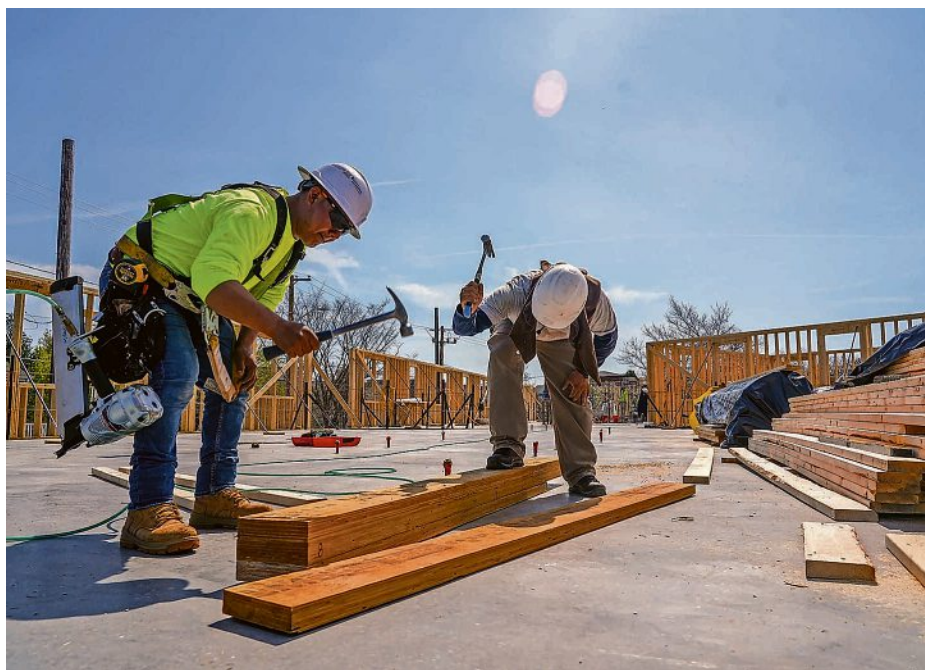
Construction of a new income-restricted apartment building is underway at the corner of Westminster and Knight streets in Providence.
