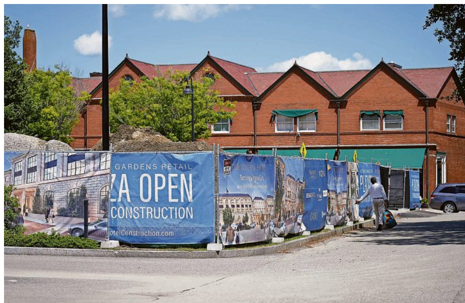
Construction is underway on the Bellevue Hotel on Bellevue Avenue in Newport, seen June 24. DAVID DELPOIO/THE PROVIDENCE JOURNAL
