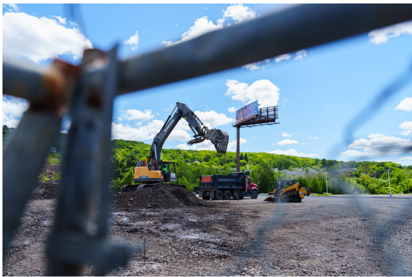
An excavator digs Monday at the site of a Wawa under construction at Moosic Street and Meadow Avenue in Scranton. The convenience store and gas station will join two existing gas stations already operating at the intersection. ISAAC DIAZ / STAFF PHOTOGRAPHER
