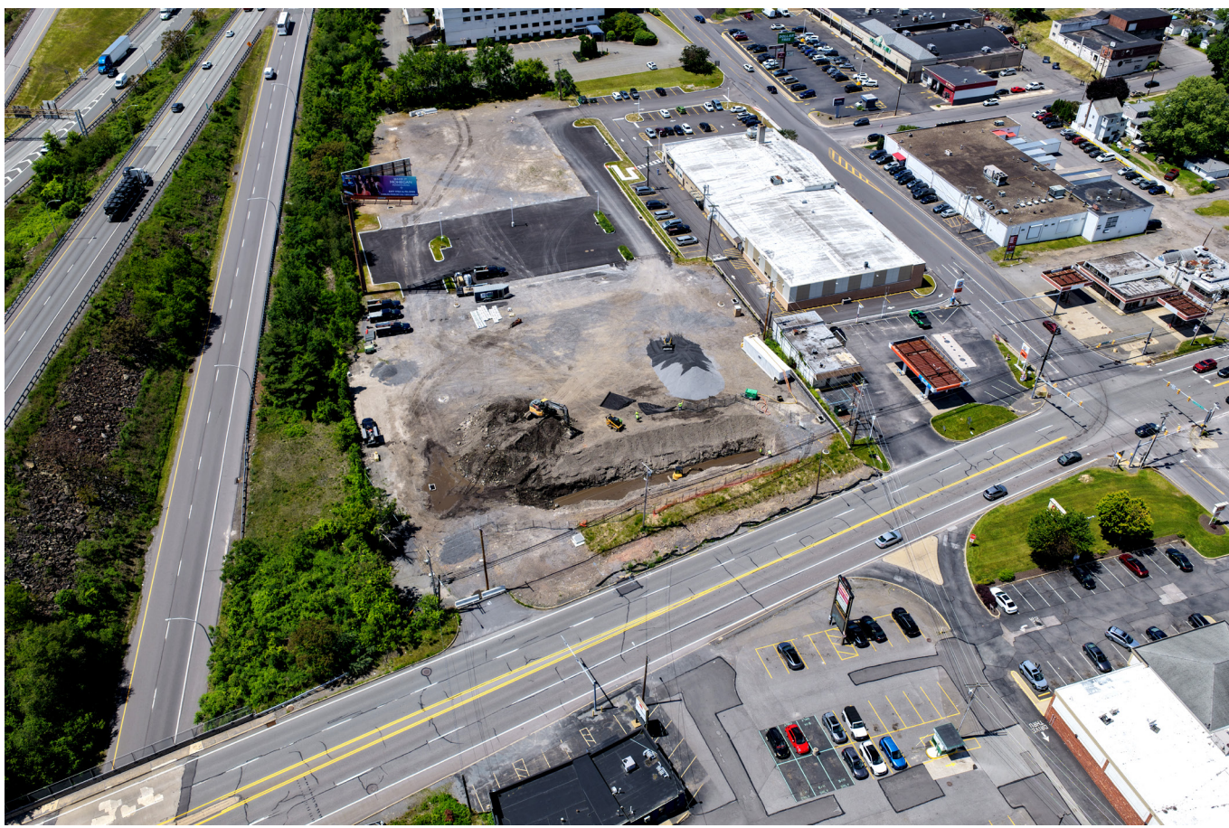
Construction is underway for a Wawa on Moosic Street in Scranton, as seen Tuesday. SEAN MCKEAG / STAFF PHOTOGRAPHER
