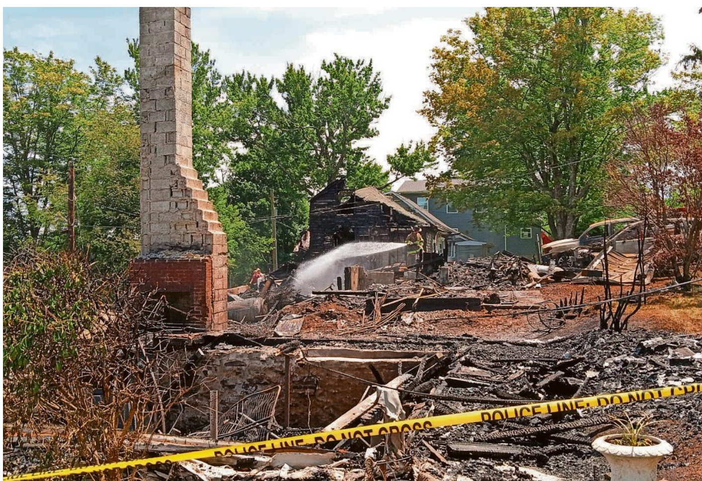
Two homes on Sensentine Road near Elk Lake in Clinton Township are leveled on June 11, after an explosion and related blaze that damaged several other houses. PETER BECKER/TRI-COUNTY INDEPENDENT
