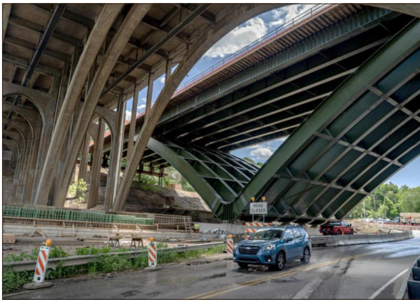
A car drives under the Commercial Street Bridge on Monday as construction work continues above. The Parkway East will close for 26 days between the Edgewood-Swissvale and Squirrel Hill exits beginning July 10.
