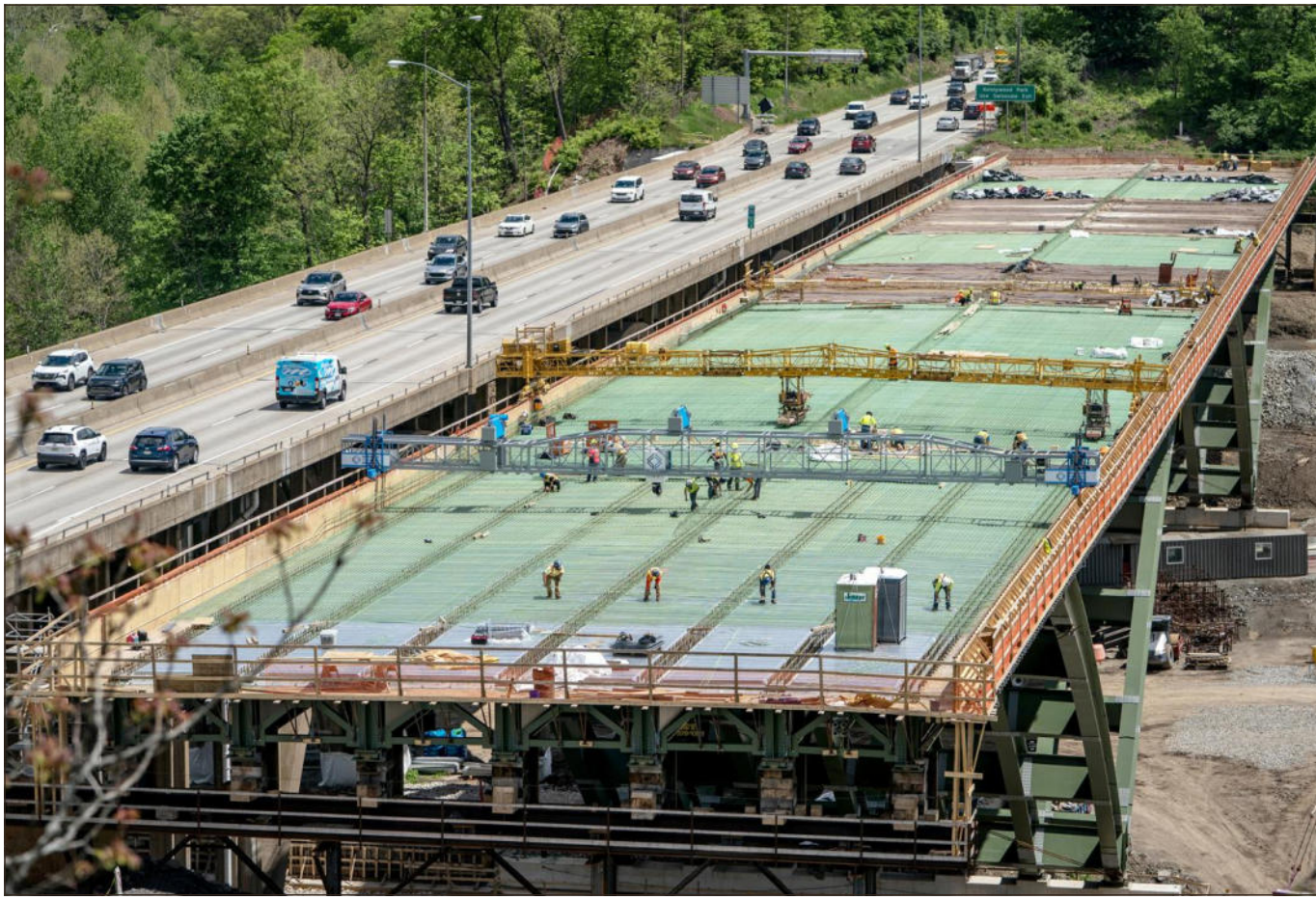
Alexandra Wimley/Post-Gazette photos As traffic passes on the existing Commercial Street Bridge, construction workers work on the bridge replacement project on Monday.
