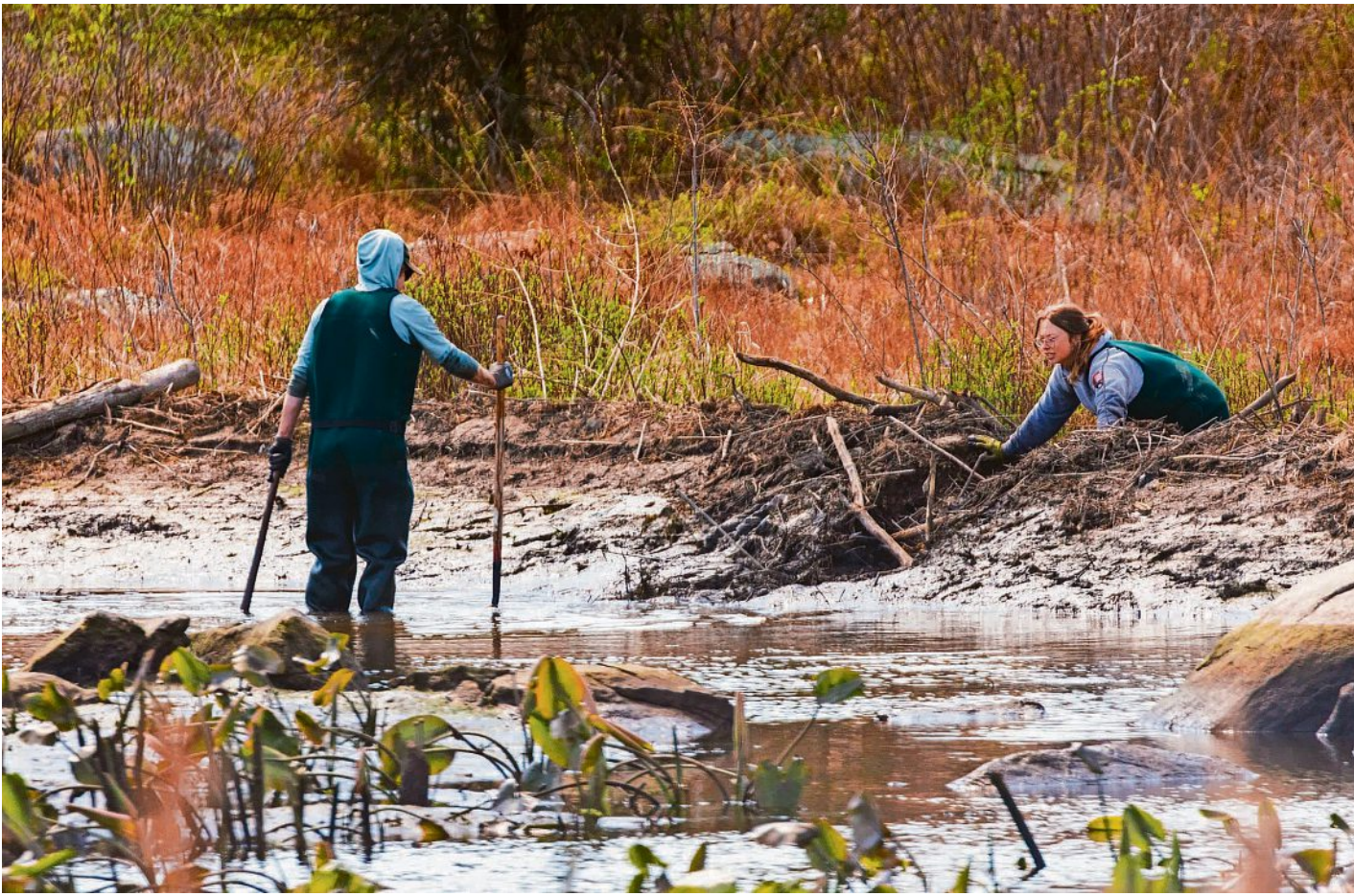
National Park Service staff work with shovels along a beaver dam during the draining of a beaver pond in Plum Run along Crawford Avenue in the Gettysburg National Military Park on Monday. HARRISON JONES/THE EVENING SUN
