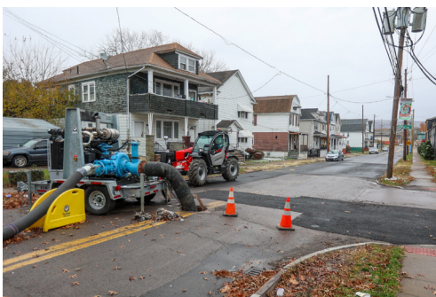
Sewer line upgrades to Horton Street in Wilkes-Barre, seen here on Nov. 11, 2025, near completion, with the street expected to be reopen to traffic by the end of the following week. THE CITIZENS' VOICE FILE
