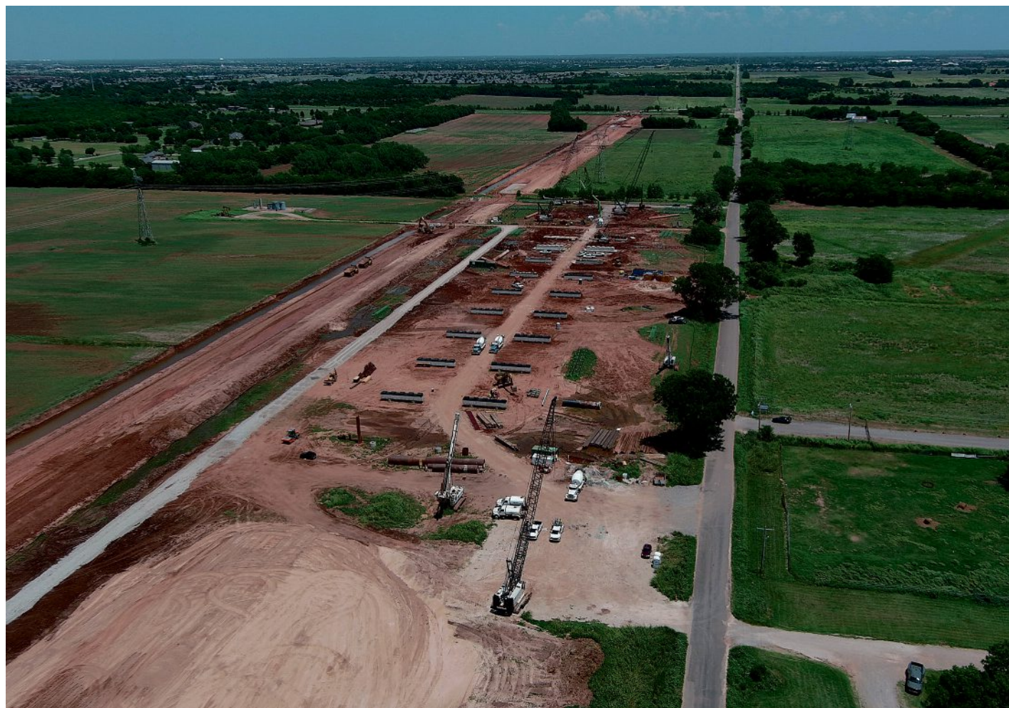
Construction is seen on July 8 on the Toby Keith Expressway in Norman. BRYAN TERRY/THE OKLAHOMAN
