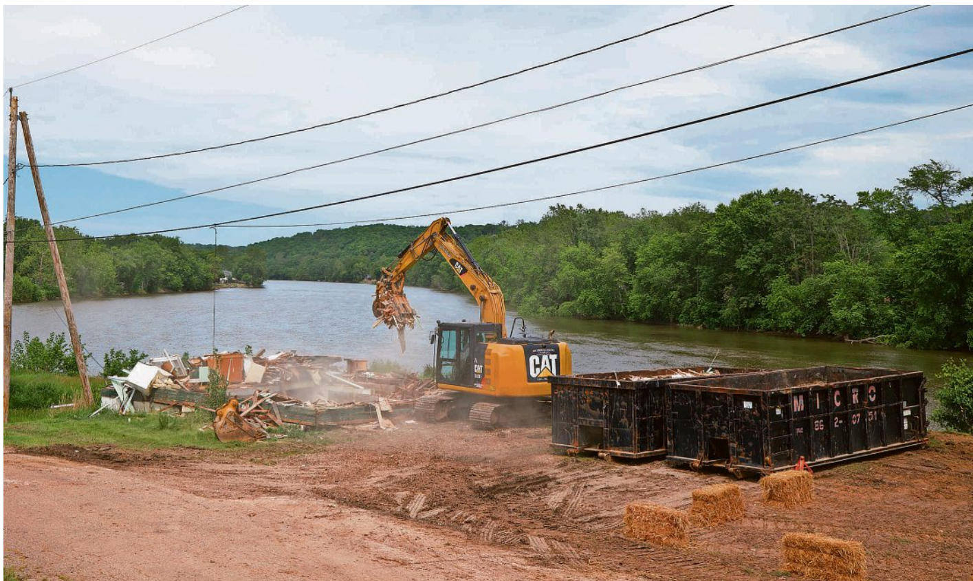
Structures near the entrance to Straker Landing have been razed. The project, spearheaded by the Muskingum Valley Park District, will rehab the former Kirkbride Marine back into an operational marina with several new amenities expected, like pavilions. SHAWN DIGITY/ZANESVILLE TIMES RECORDER
