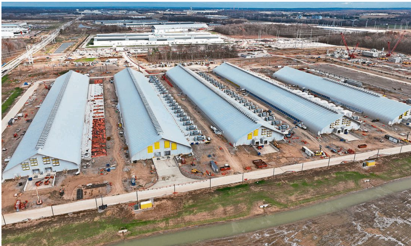
Five tents holding Meta AI data centers for Facebook are under construction in New Albany photographed Nov. 28, 2025. DORAL CHENOWETH/COLUMBUS DISPATCH
