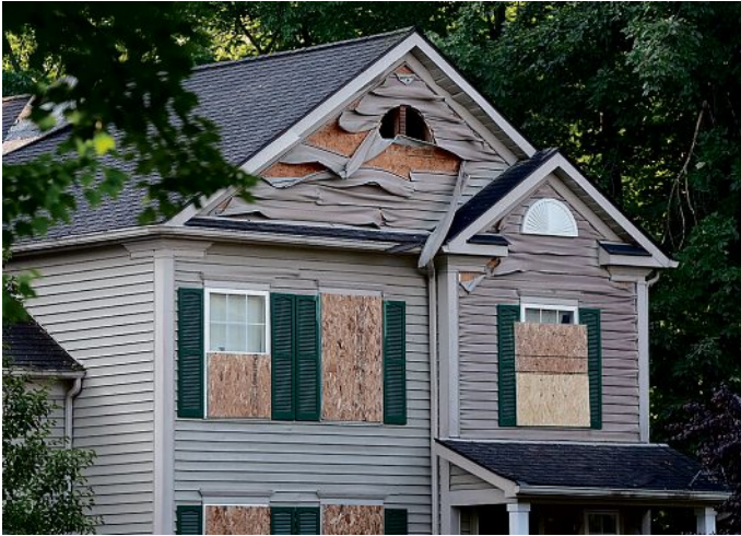
After the Twinsburg gas explosion last month, residents and officials are questioning how fiber optic cable is being installed underground. Here, the siding on a home on Hiram Lane in Twinsburg Township melted from the heat of the explosion.
