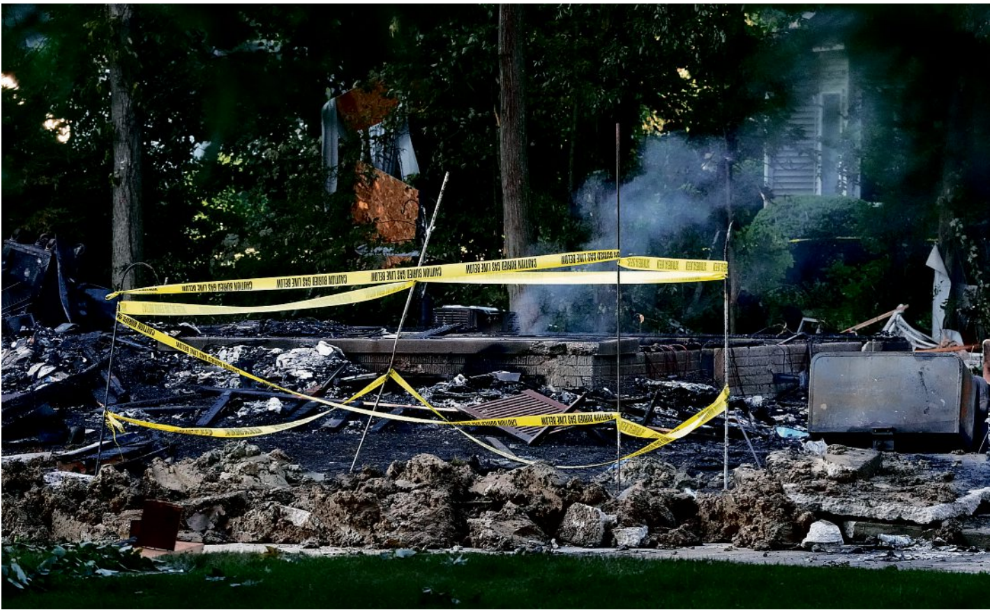
Contractors hit a gas line in Twinsburg Township on June 25. The gas line rupture and explosion destroyed three homes and damaged 36 others. PHOTOS BY MIKE CARDEW/AKRON BEACON JOURNAL
