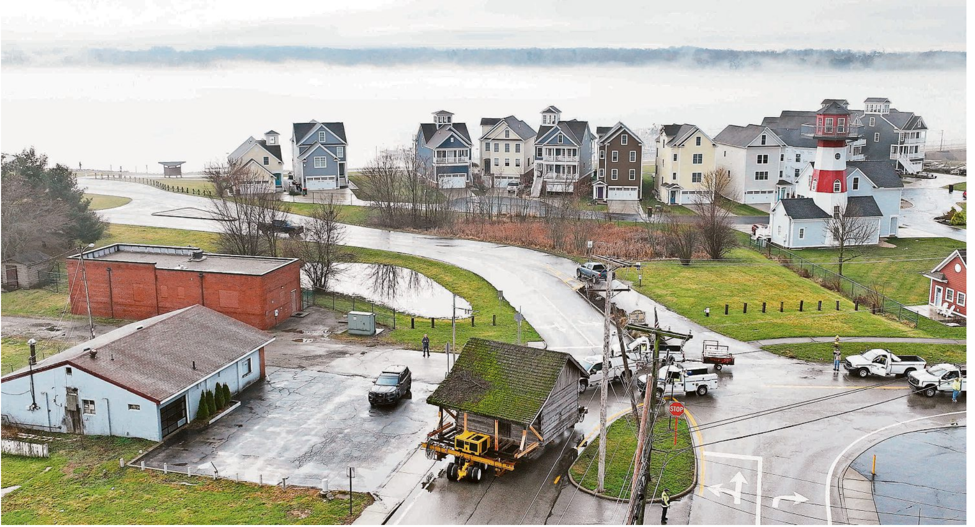
Crews from Dingey Moving, the village of Buckeye Lake, Spectrum, American Electric Power, Ohio Department of Transportation and others move the Historic Holtsberry Log Cabin on March 6 to village-owned property at 10500 Mill Dam Road. The cabin dates back to 1820, and the move aims to preserve it for future generations. DORAL CHENOWETH/COLUMBUS DISPATCH
