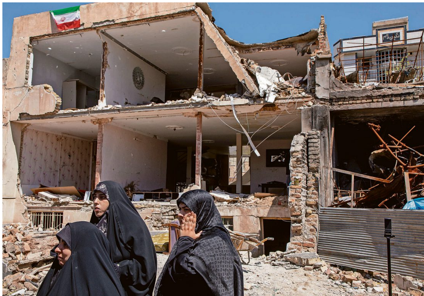
People stand outside a damaged residential building April 3 in Karaj, Iran. AJID SAEEDI/GETTY IMAGES
