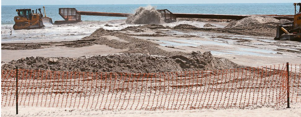
A South Jersey beach undergoes restoration work here as part of a 2015 U.S. Army Corps of Engineers project. PHOTOS PROVIDED BY U.S. ARMY CORPS OF ENGINEERS
