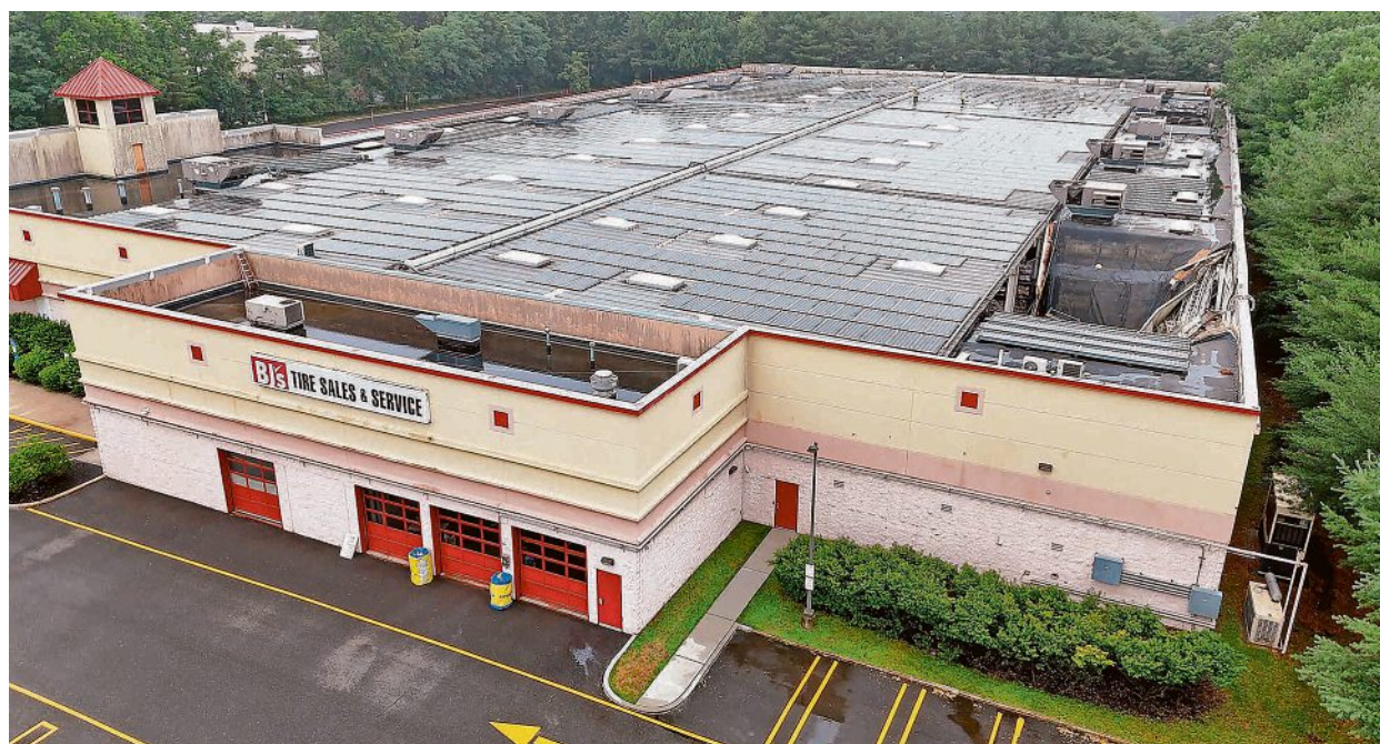
A collapsed portion of the roof at the BJ's in Ocean Township is shown Monday afternoon, July 6. Heavy rains had swept through the area and caused numerous incidents of flooding and downed trees.
