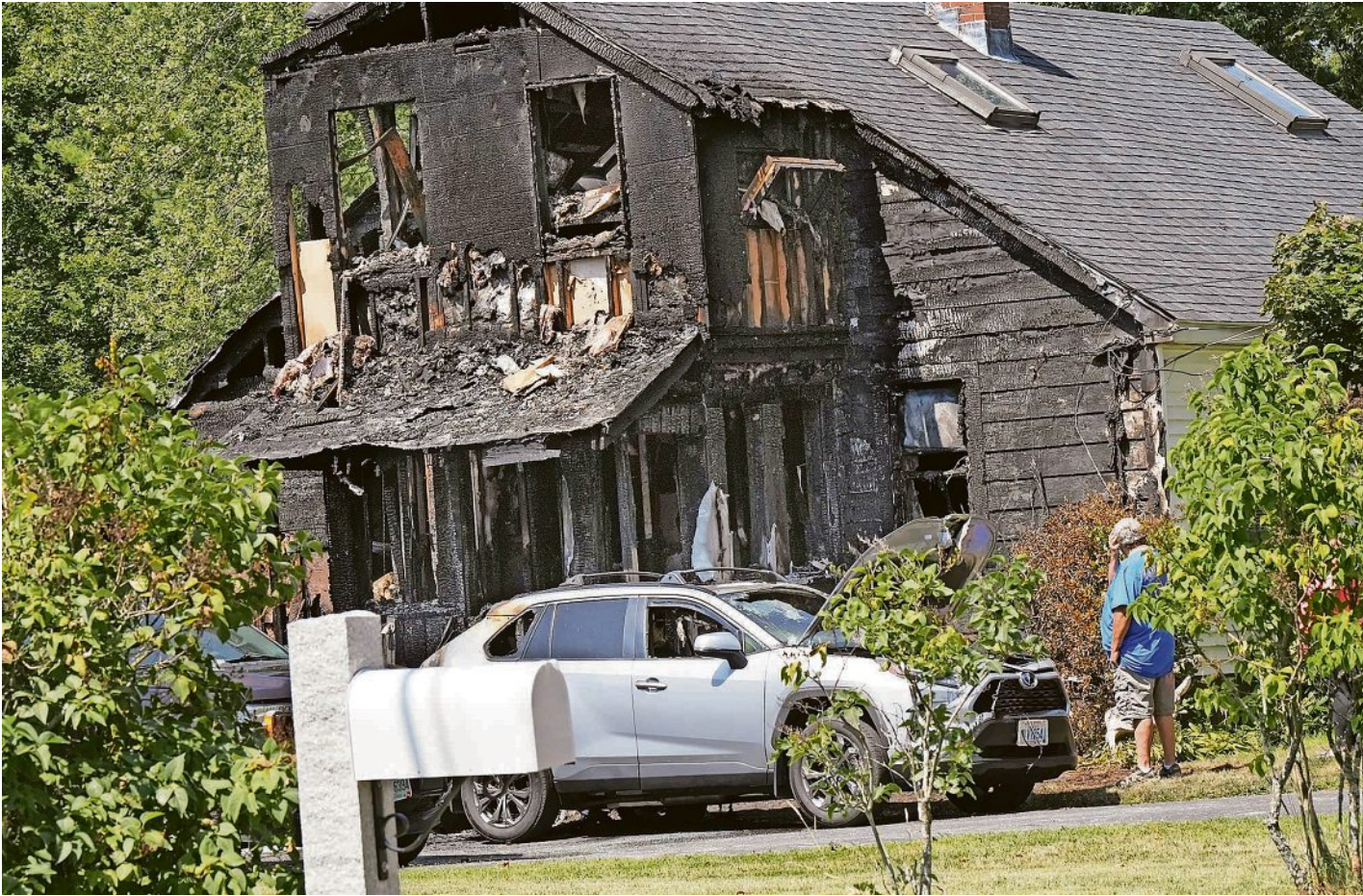
Heavy damage is seen from a fire at 14 Old Rochester Road in Dover Aug. 16. DEB CRAM/FOSTER'S DAILY DEMOCRAT
