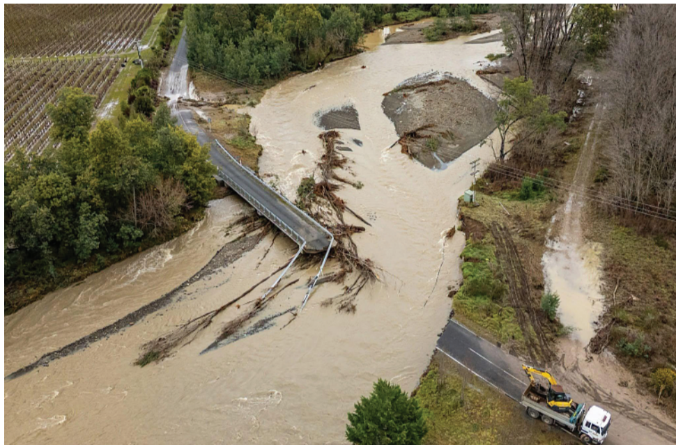
The Tyntesfield bridge, in Marlborough's Waihopai Valley, has been destroyed this week by a raging river. Flooding will cause greater damage to road networks in future. GAVIN HADFIELD
