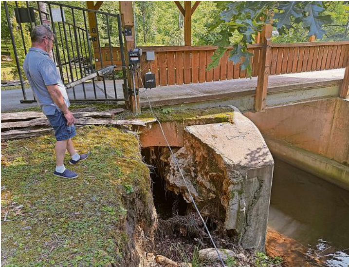
Marc DiFrancia inspects damage to his bridge caused by Tropical Storm Helene in 2024 in Candler. As of July 1, it was only getting worse. CORY VAILLANCOURT/ASHEVILLE CITIZEN TIMES
