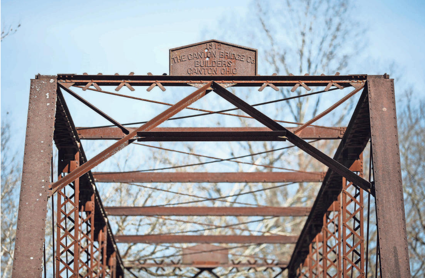
The 112-year-old Green Bridge, which crosses the Finley River near Ozark in Christian County, has been closed by the Missouri Department of Transportation after an inspection rated the bridge a 2 on a 10-point scale.
