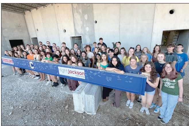
Carthage High School choir, band and drama students took some time out of their summer Tuesday to put their names on the last structural steel beam that will be put in place in the Carthage High School auditorium, which is scheduled for completion in the summer of 2027. GLOBE | JOHN HACKER
