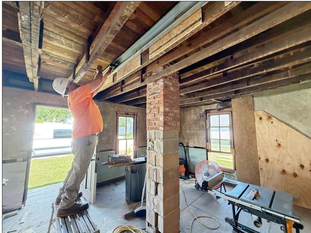
Chris Goodfellow, site supervisor working on the Neosho Colored School, measures floor joists for the attic to add steel reinforcing beams.
