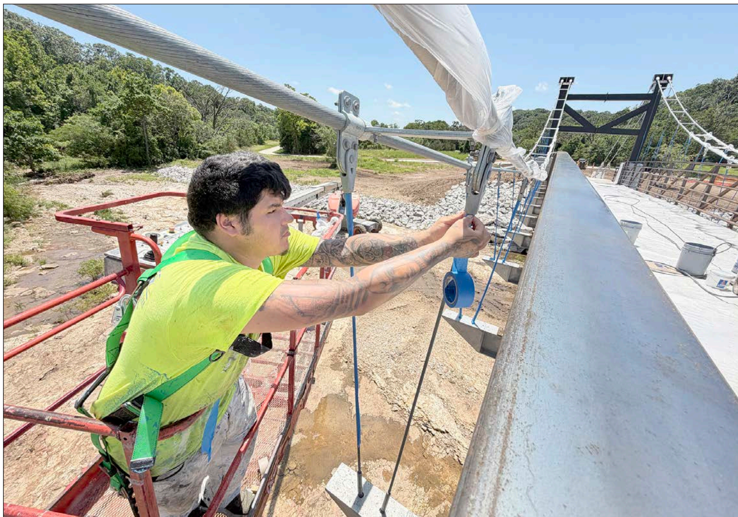
Alejandro Acevedo, of Webb City, with Evans Painting, surrounds cables on the new Tin Cup Trail suspension bridge with tape as the bridge is being readied for painting Wednesday.
