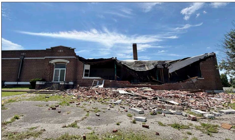
A storm caused extensive damage to many buildings in the area Saturday night and Sunday morning, including the former Eugene Field Elementary School in Carthage, which recently served as a church.
