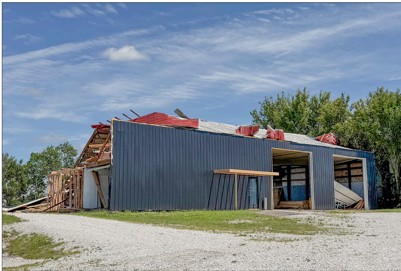
The building housing JB Electric at 120 N. Prigmore Ave. in Duenweg was badly damaged in the storm over the weekend.
