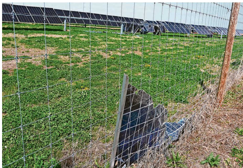
This section of the Apex Coldwater solar farm was taken offline for repair after less than two dozen panels were damaged by the April 15 tornado.
