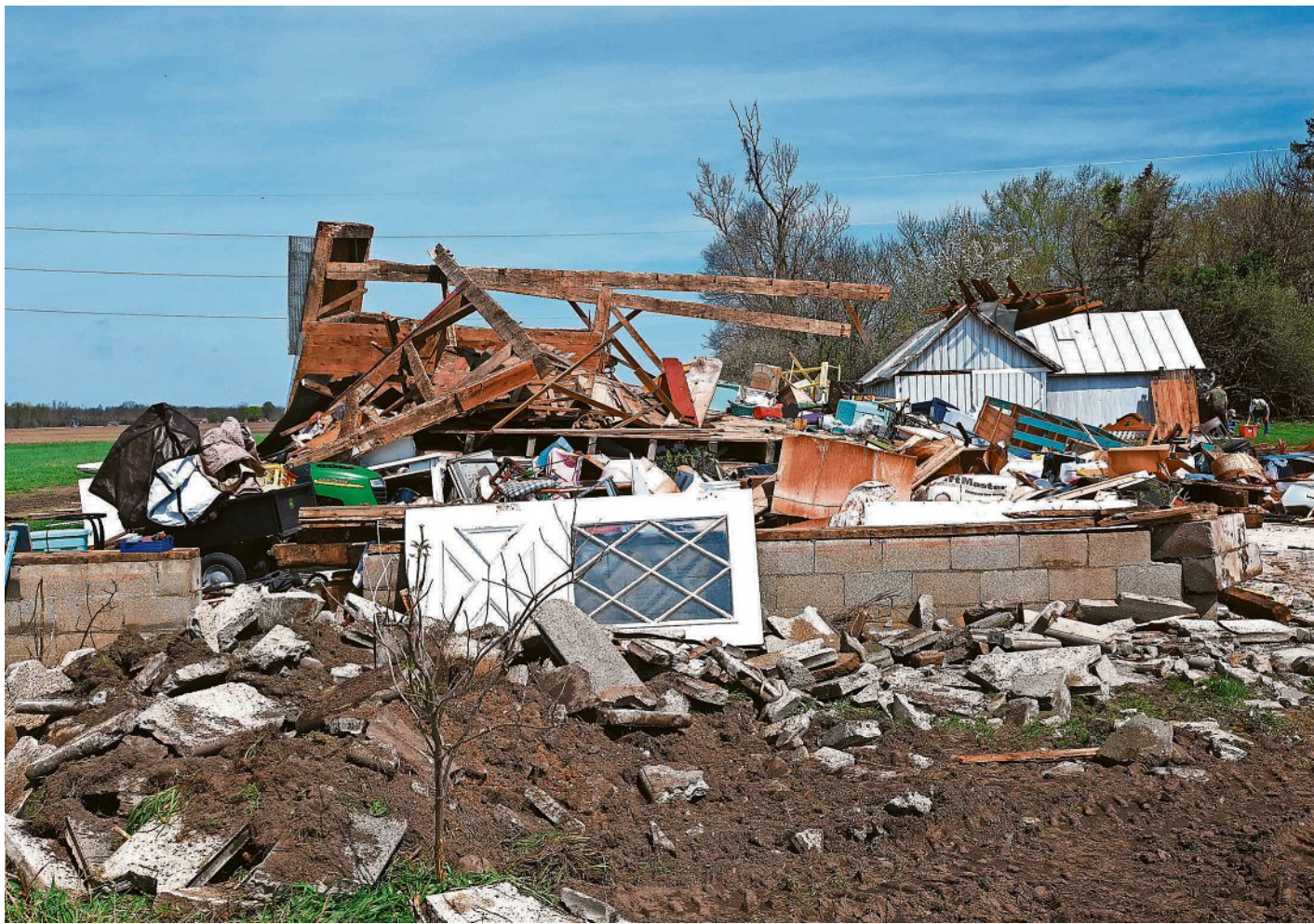
Part of this historic 1860s barn was torn off and dropped on the roof of the nearby pole barn off Sanford Road by the April 15 tornado. PHOTOS BY DON REID/COLDWATER REPORTER
