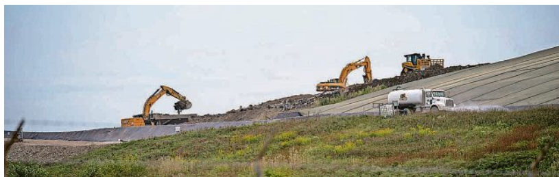
A backhoe fills a dump truck at the Wayne Disposal Inc. hazardous waste landfill in Wayne County's Van Buren Township. MANDI WRIGHT/DFP
