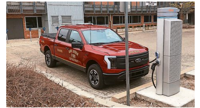
An all-electric Ford F-150 Lightning used by the city of Ann Arbor charges at Ann Arbor's city hall. The city is working to launch a new program that will pay rebates to residents who buy EVs. PROVIDED BY ANN ARBOR OFFICE OF SUSTAINABILITY AND INNOVATIONS
