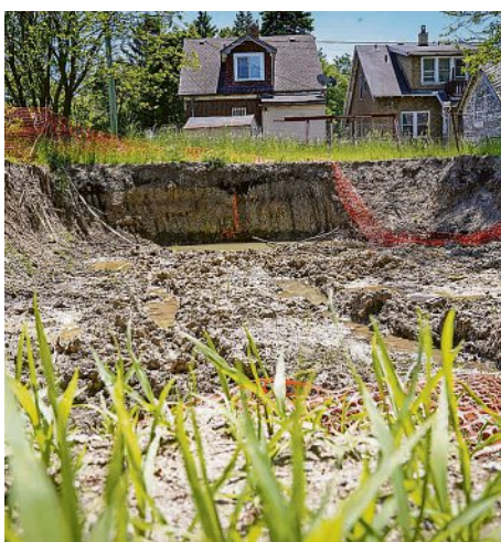
An excavated lot is seen at 8070 Wisner in Detroit on May 28. Soil tests ordered by the Detroit Office of the Inspector General found excessive contamination at the lot, where contractor Gayanga previously demolished a home.
