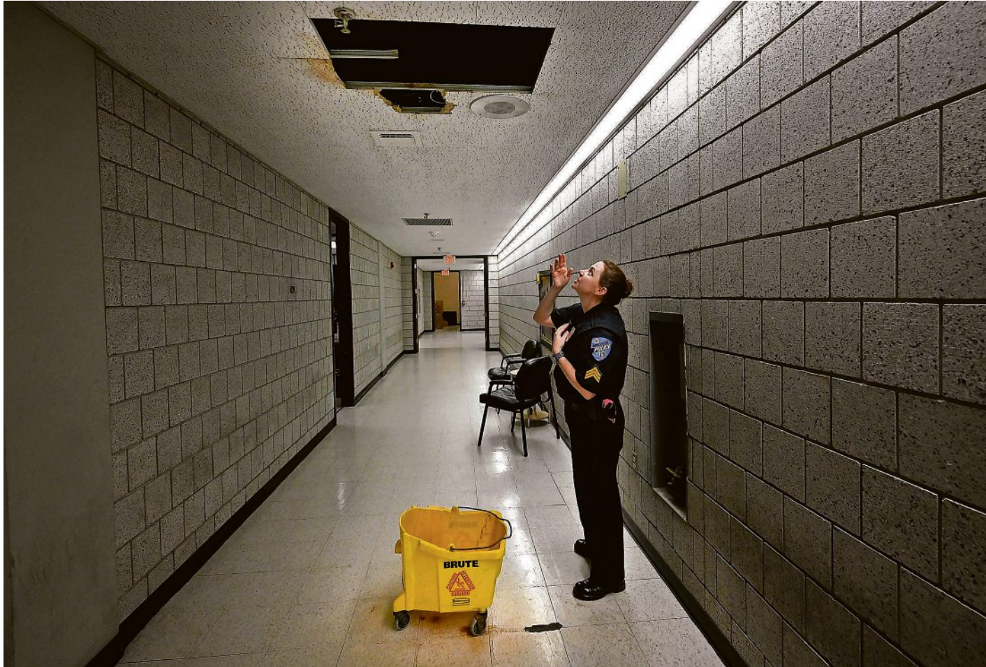
At Worcester Police Department headquarters, Sgt. Elise B. Miranda stands near a mop bucket collecting water under a leak in the third-floor hallway outside the Bureau of Professional Standards. PHOTOS BY ALLAN JUNG/TELEGRAM & GAZETTE
