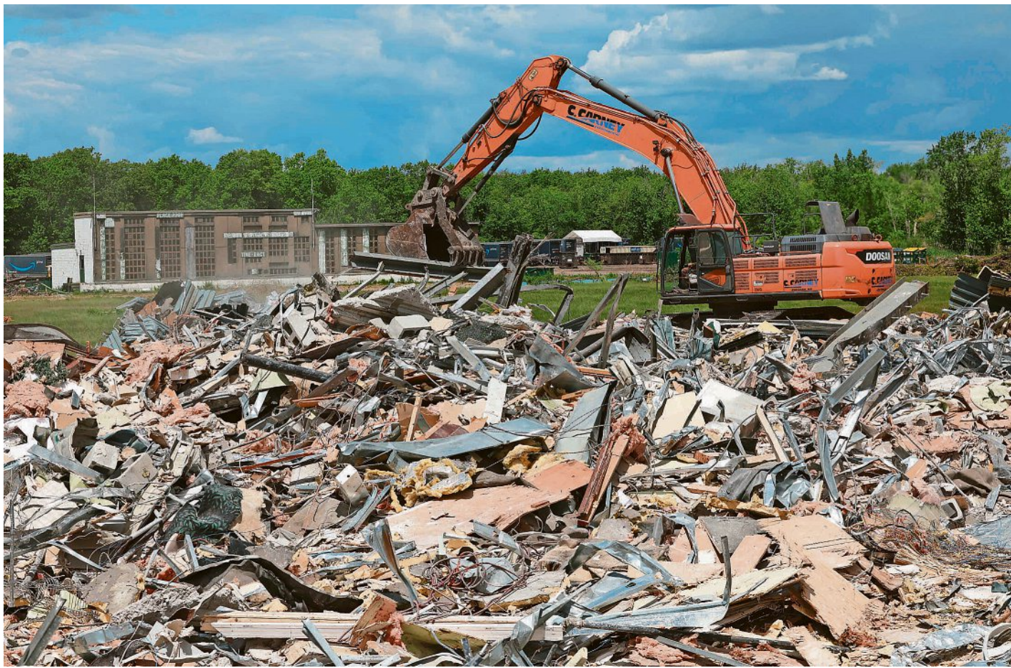
Raynham Park is seen May 28 as the clubhouse was demolished. PHOTOS BY MARC VASCONCELLOS/THE ENTERPRISE
