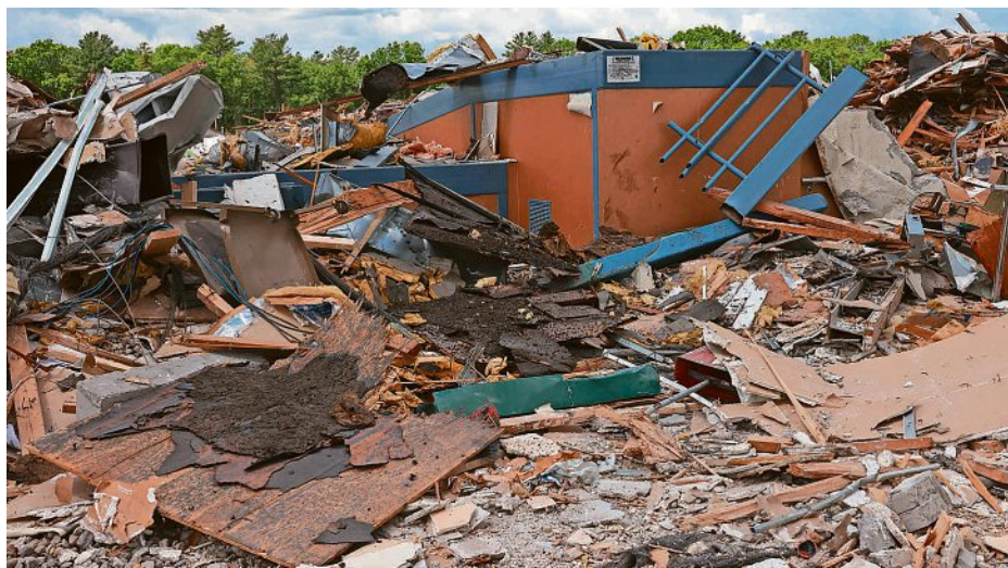
The entrance to the clubhouse was demolished at Raynham Park on May 28.
