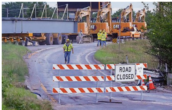
Huge steel beams are moved into place on June 1 as construction begins on I-65. The on ramp is at Shelby Street. MICHAEL CLEVINGER/COURIER JOURNAL
