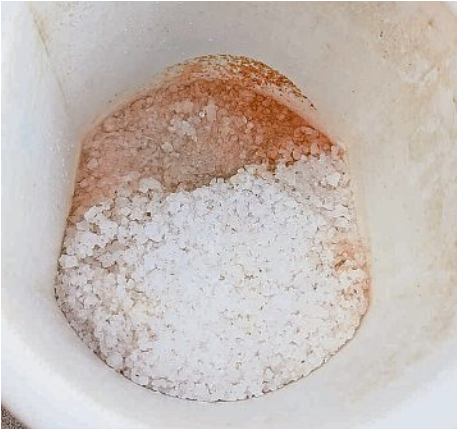
Salt from Linda Close's water softener has turned brown in her system. Close believes this same water is causing damage to her washing machine, water heater and other appliances.
