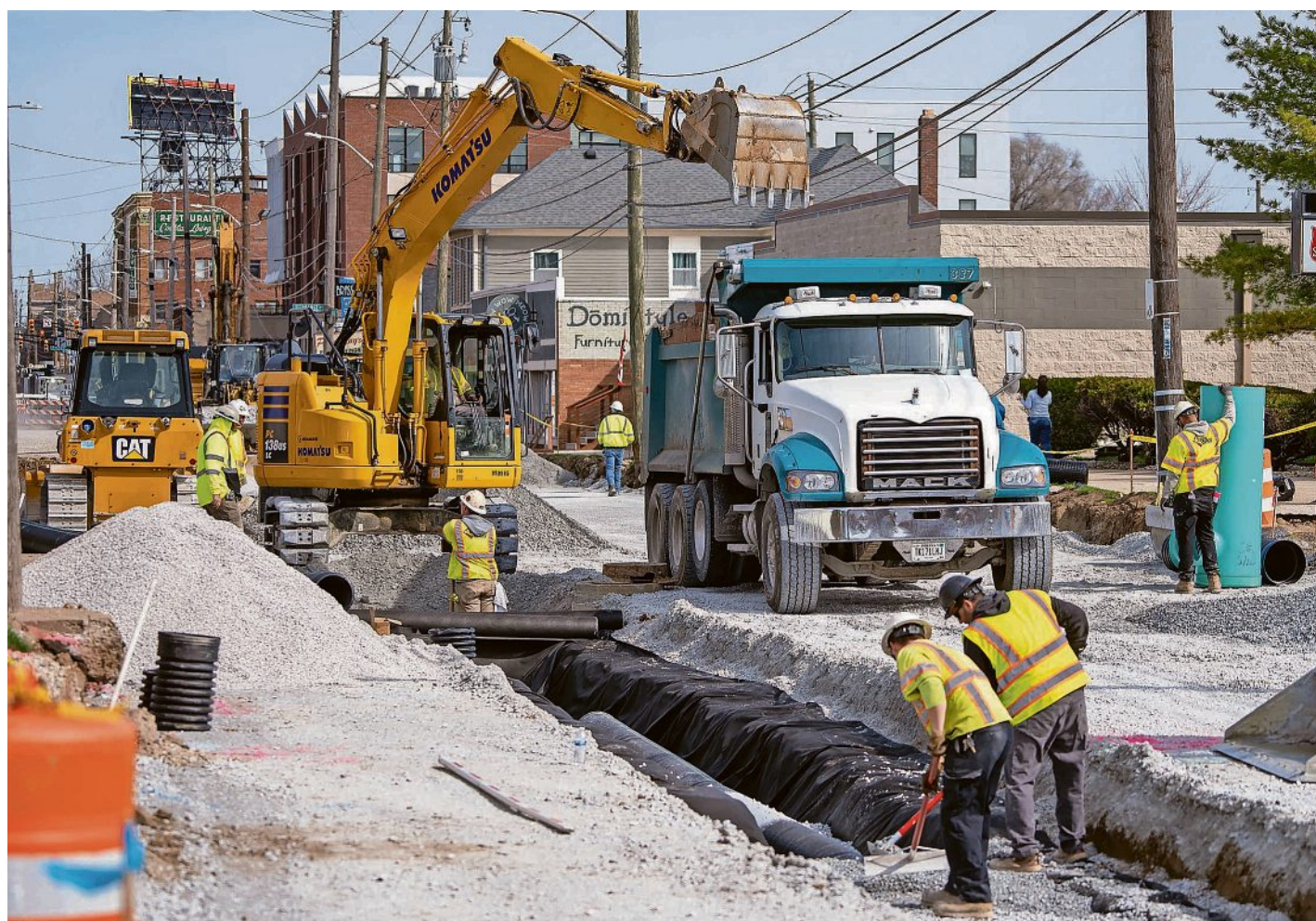
Construction continues March 25 along Shelby Street in the Fountain Square area of Indianapolis.
