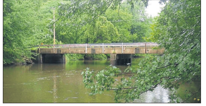
Photo provided / Elkhart County Highway Department Pictured is Bridge No. 332 ahead of emergency repairs carried out last year.
