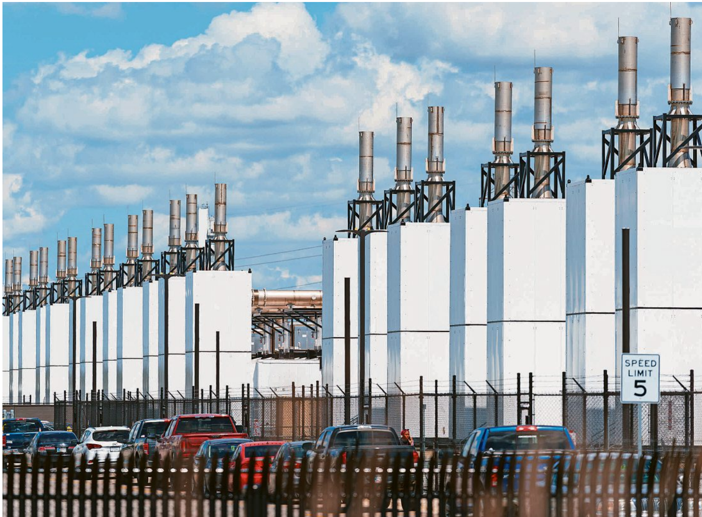
Project Rainier, an $11 billion Amazon AI data center is pictured on April 23 between New Carlisle and South Bend.
