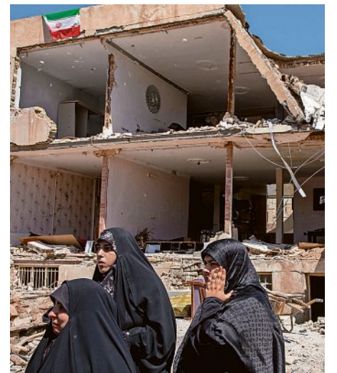
People stand outside a damaged residential building April 3 in Karaj, Iran. AJID SAEEDI/GETTY IMAGES
