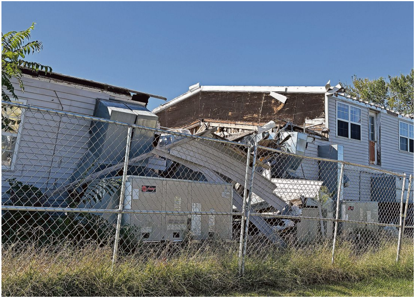
Damage to Animal Protective League’s shelter building from a June 10 EF-1 tornado is pictured here Oct. 4. The shelter building, a former campground, and another building formerly used to spay and neuter cats and dogs, will be demolished. PHOTOS BY STEVEN SPEARIE/THE STATE JOURNAL-REGISTER
