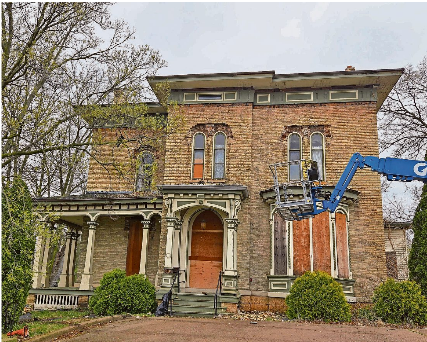
UW Health has acquired several properties seen Monday including Rockford's Briggs Mansion, 1244 E. State St., in addition to 1238, 1246, 1250 and 1318 East State St., with plans to demolish them in May and make way for a SwedishAmerican Hospital future expansion project. JEFF KOLKEY/ROCKFORD REGISTER STAR
