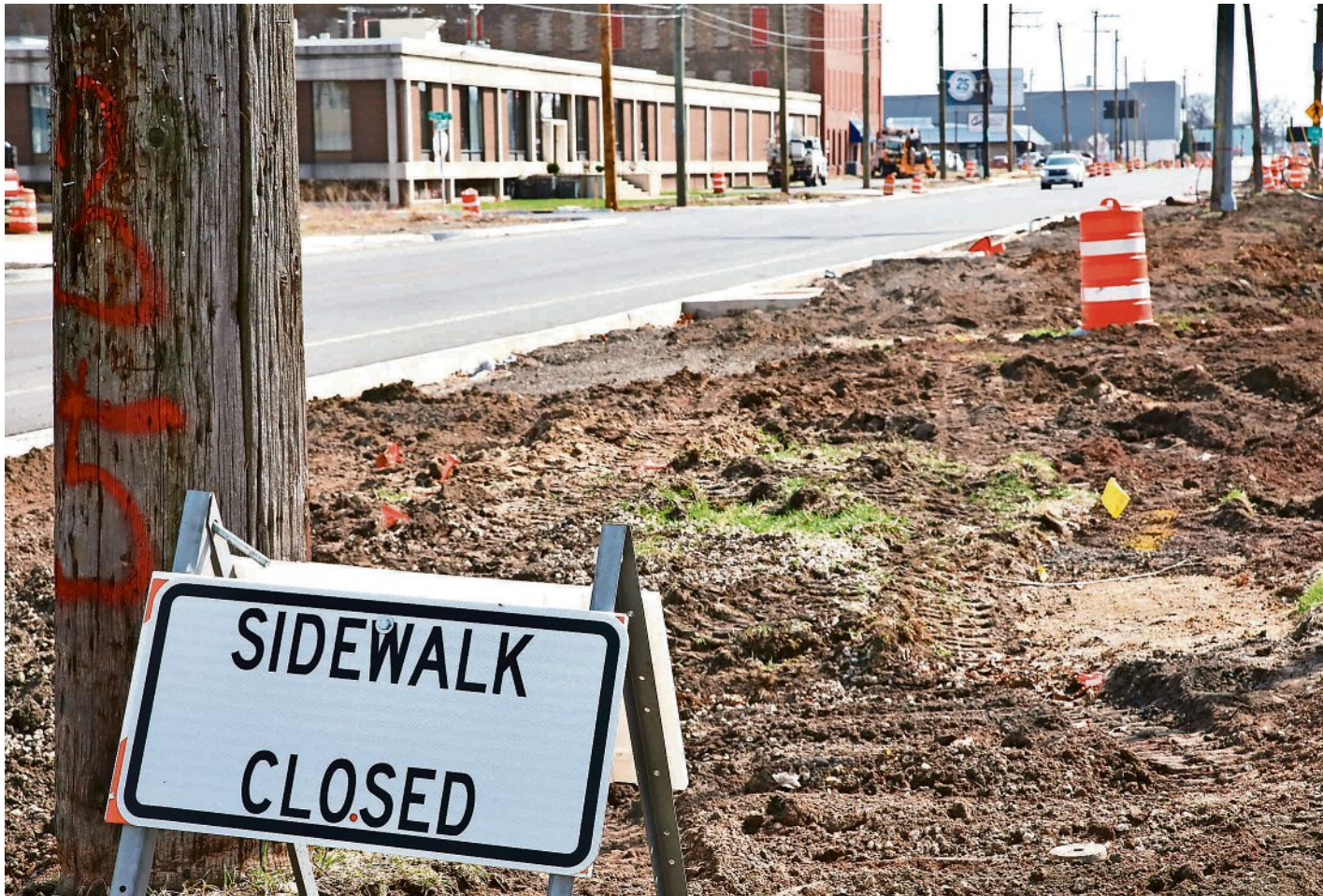
Undergoing a $29.2 million multi-phase reconstruction, 11th Street is pictured near 22nd Avenue on March 25, heading south in Rockford. PHOTOS BY SUSAN MORAN/ROCKFORD REGISTER STAR
