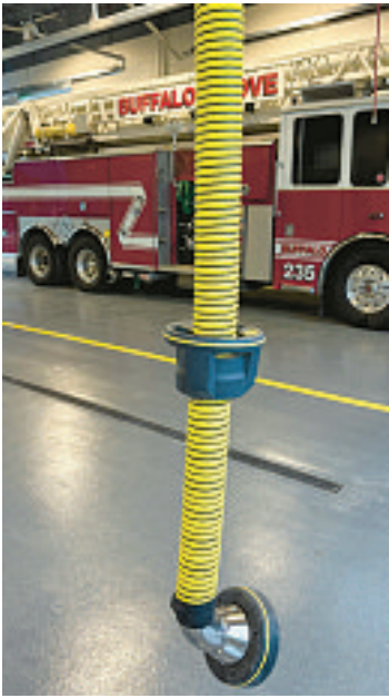
The new fire station has a hose that extracts vehicle exhaust and vents it outside the station.
