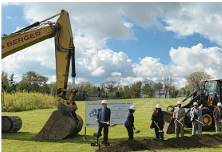
Local officials break ground on the Lewis Avenue detention basin in North Chicago, which will be a passive park most of the time. CITY OF NORTH CHICAGO
